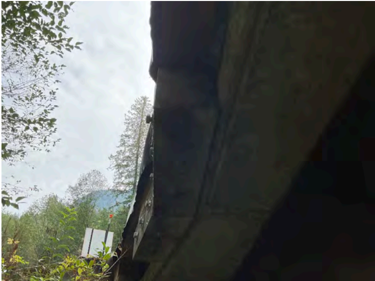
Loose rail hardware
