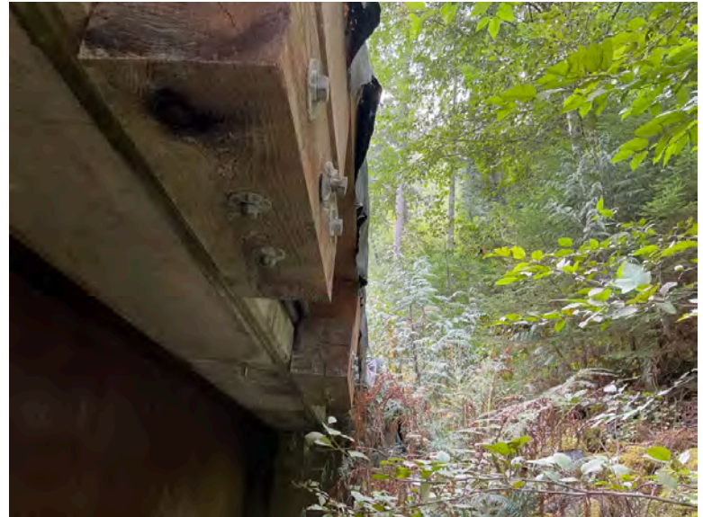
Loose rail hardware
